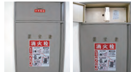
Emergency telephones and indoor fire extinguishers (Center Bldg.)
